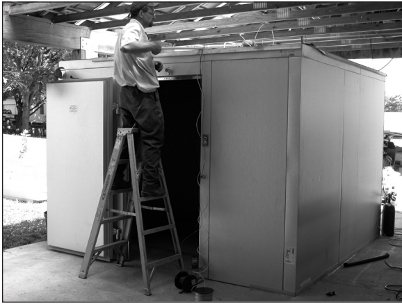
Installation being done by Vince Kling and Jim Nolt from Rufus Brubaker Refrigeration, Manheim.
