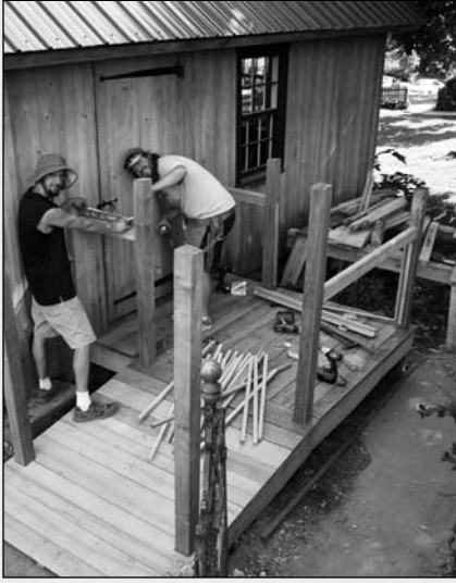
Kirk Hawthorne and Ben Krouse construct a wheelchair-accessible ramp to the new office.
